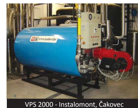
VPS 2000 - Instalomont, Čakovec
